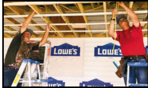
Group 1: Rob Hunt and Robert Massery work on wiring for Auxier porch
