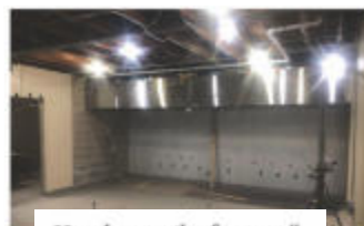
Hoods over the fryer wall
