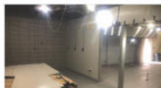
Electrical outlets in serving room
