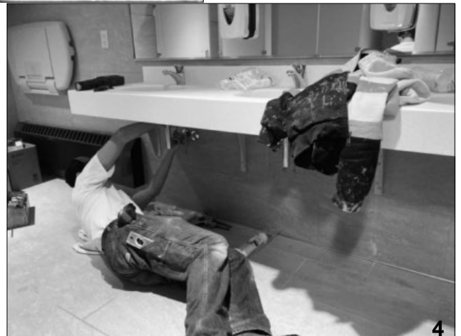
Below: Plumbing being worked on in bathrooms hooking up sinks and toilets.
