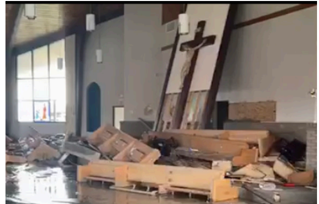
Hurricane damage to Our Lady Star of the Sea Catholic Church in the Diocese of Lake Charles Louisiana
